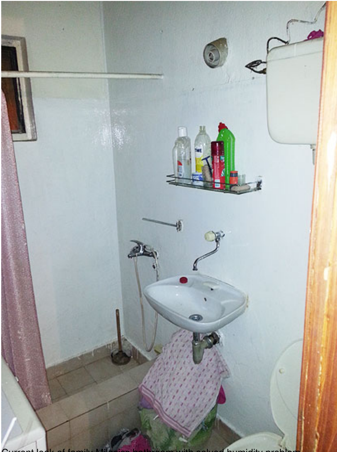
Current look of family Milacics bathroom with solved humidity problem
